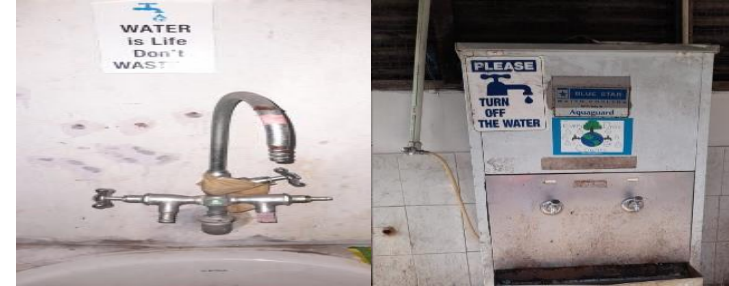
Instructions to turn off the water taps after use
