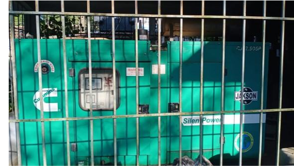
DG Set for Power Back up
